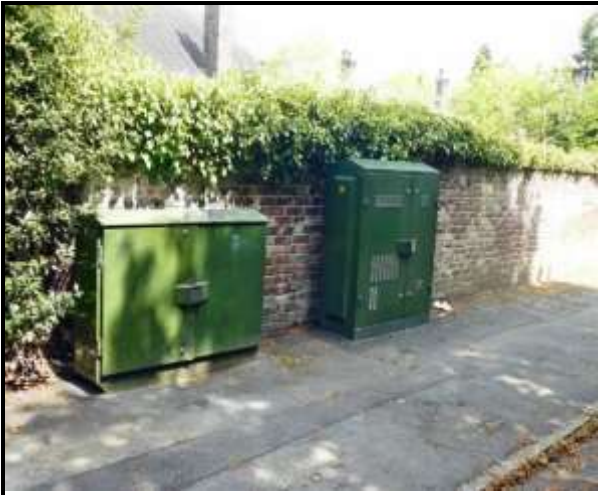
Photograph 26: Services Cabinets, Booth Road
