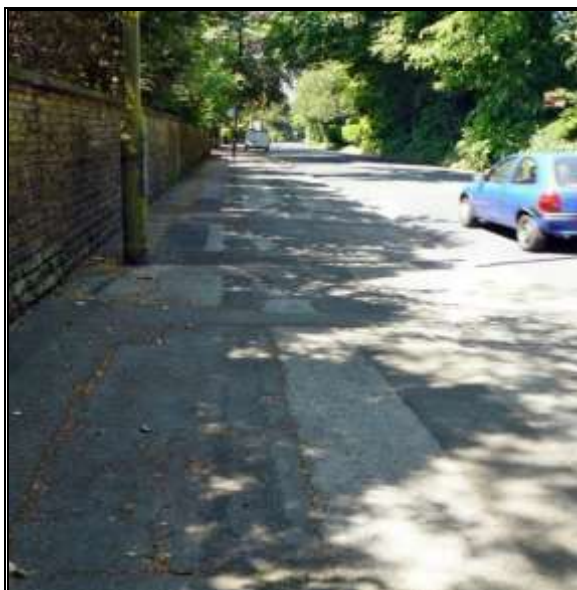
Photograph 129: Example of Patch Repairs, Park Road
