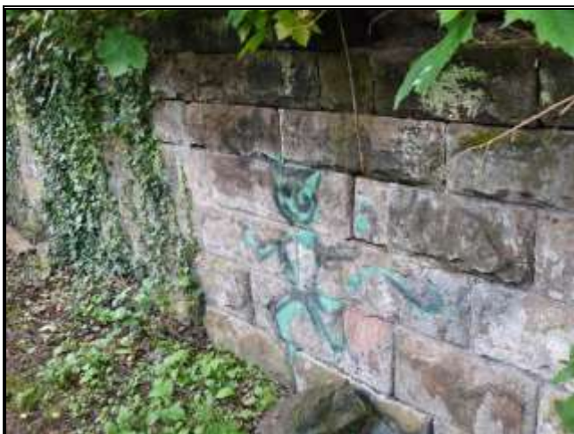
Photograph 131: Graffiti along Passageway in Character Zone A
