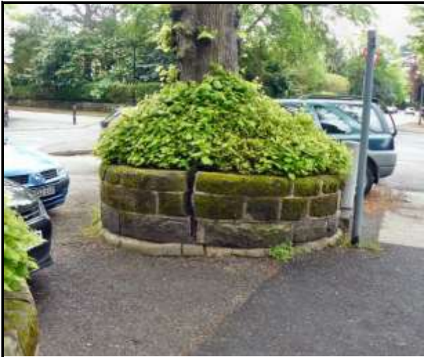
Photograph 119: Cracked Stone Planter, St Marys Road
