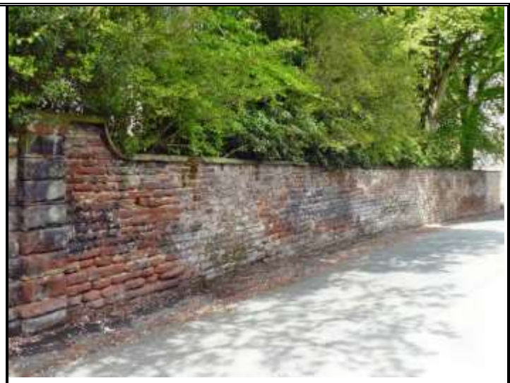
Photograph 118: Damaged Stone Boundary Wall along Gorsey Lane
