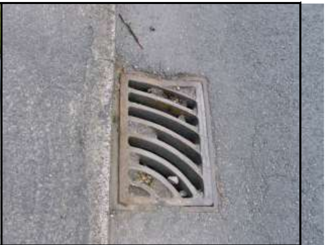
Photograph 101: Drain Cover, Charcoal Road
