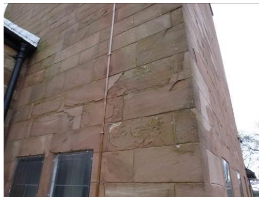
Delaminated sandstone to church tower
