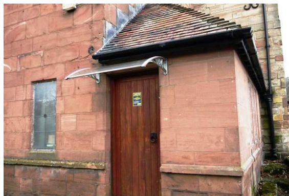
Inappropriate detailing on the church
