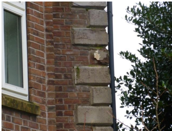
Delaminated stone quoin to Old Hall Farmhouse
