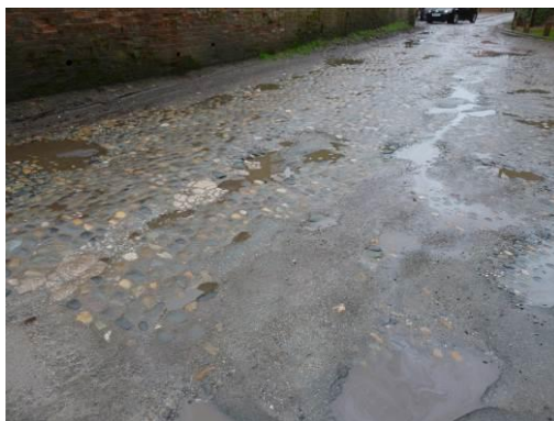
Uneven and partially covered stone sett surface
