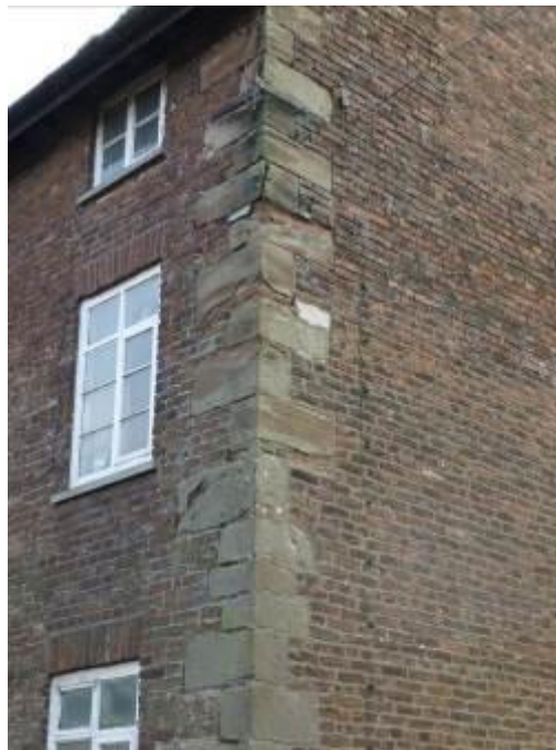
Eroded Quoins to Little Heath Farm House
