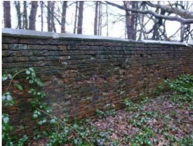
Section of estate wall with eroded pointing, spalled bricks and damaged copings
