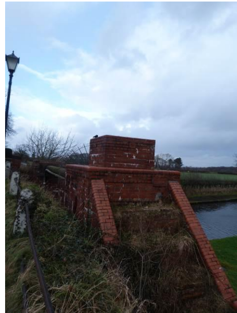
Elevated pipeline by Dunham School Bridge
