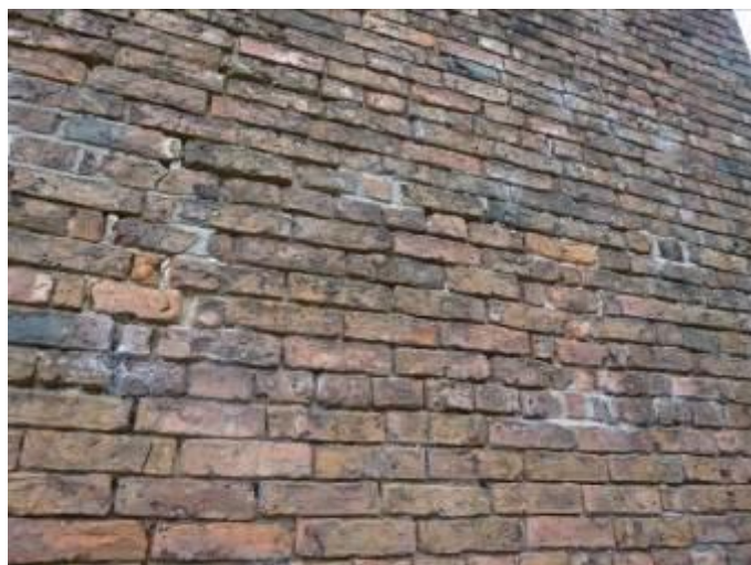
Eroded pointing to the barn at Big Tree Farm
