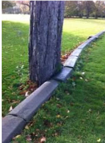
Large tree adjacent to ha-ha wall, forcing masonry out of line
