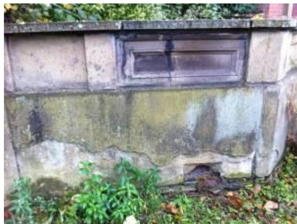
Delaminating masonry to the plinth walls of Longford Hall
