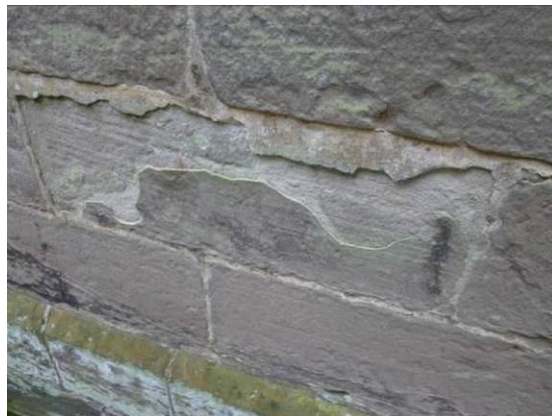
Example of delamination to ashlar on St. Werburgh's Church
