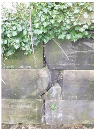
Crack and vegetation to bridge balustrade wall
