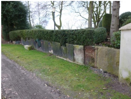
Vertical sandstone flag boundary wall to rectory, with multiple fractured flags
