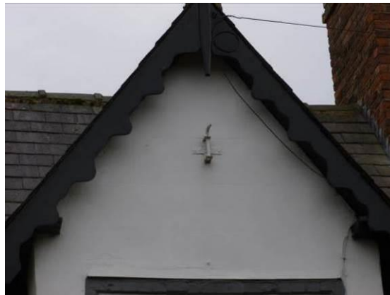
Incised joints to render of No.4 Church Green dormer gable
