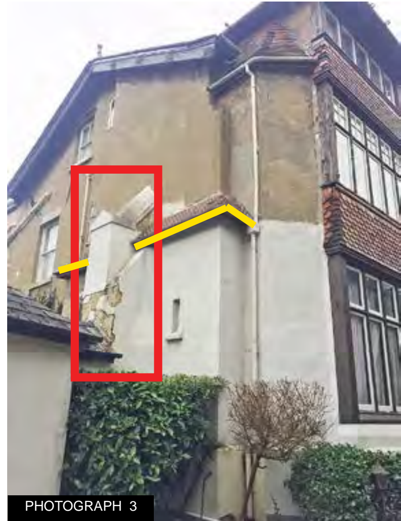
The strange buttress edged in red may have been added to help support the projecting bay on either side of the full height chimney breast indicated by the yellow line. It may explain why the stack above gable level was demolished.
