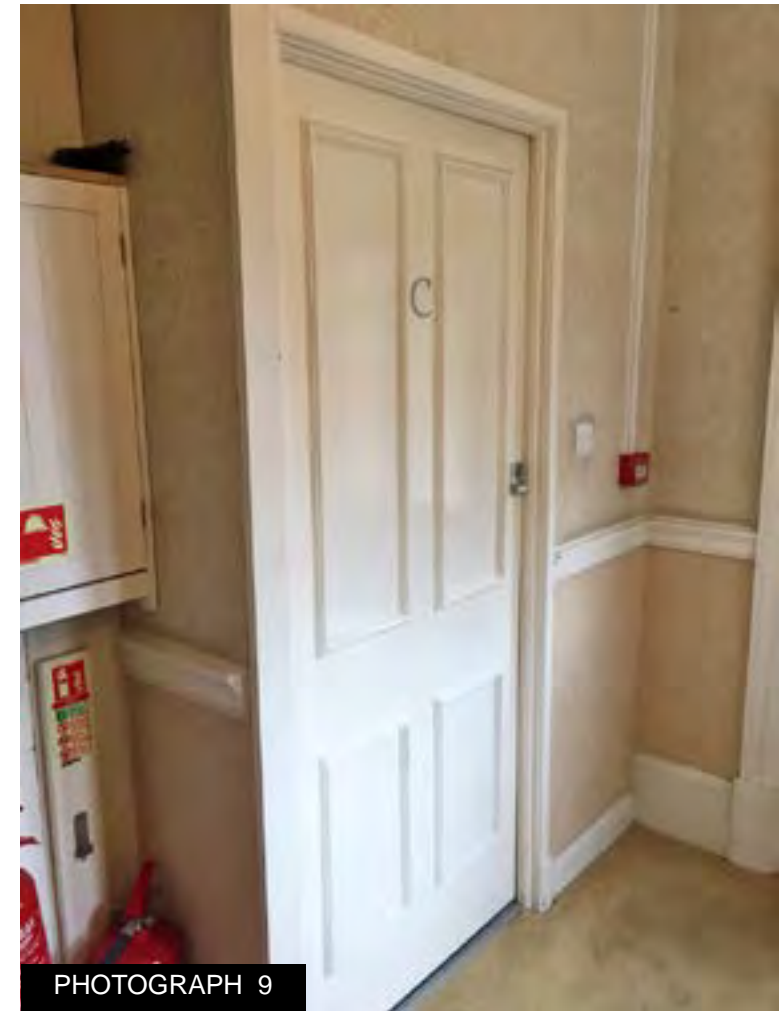
Entrance to one of the GF flats created off the main hallway. Note the contrast in the height between the old and new skirting boards.
