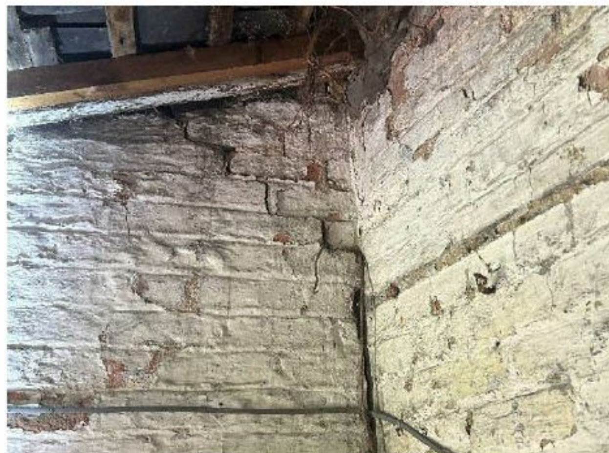
Plate 6 - Gaps in brickwork in Building 5.
