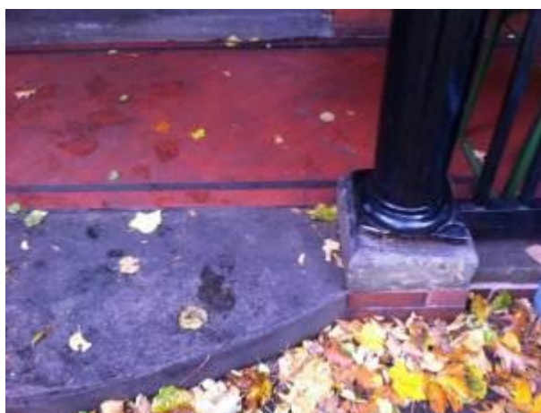
Damage to base of timber column by main entrance
