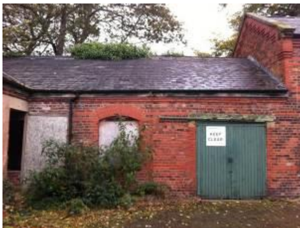
Slipped slates, damaged gutters and vegetation to former stables
