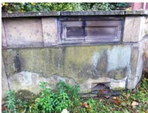
Delaminating masonry to the plinth walls of Longford Hall
