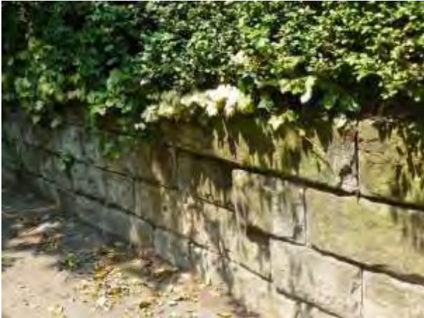
Damaged wall on Harrop Road
