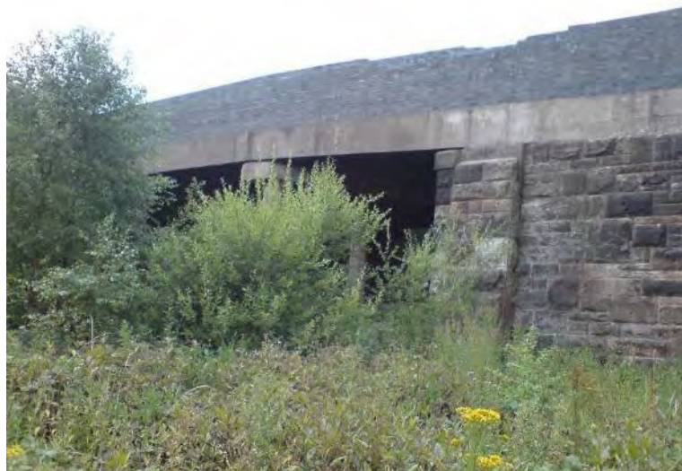
Figure 49 - Missing brick to parapet (over span 1)
