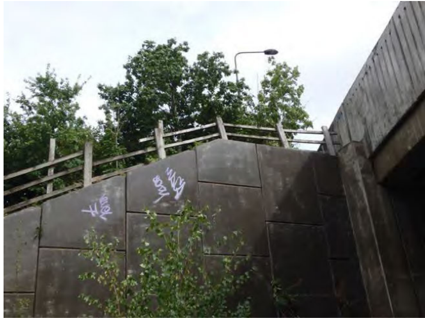
Figure 55 - Damaged and unstable fences above wing walls
