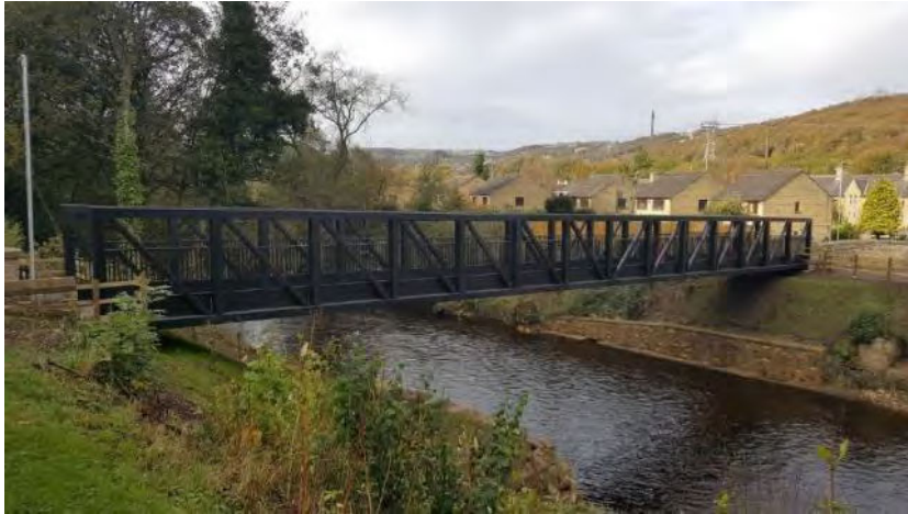
Figure 58 - Photo showing a Pratt truss of similar form, although this structure only carries a footway/cycleway. Option 1 requires a slightly heavier structure with 1.8m parapets to carry equestrian and maintenance vehicle loading
