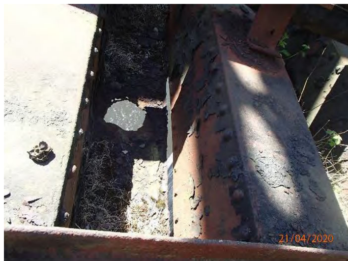
Figure 57 - Typical example of the more severe corrosion damage to trough decking. Note the complete loss of section at the bottom of the trough (typical)
