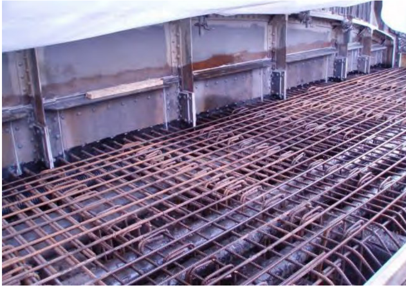
Figure 60 - Photo showing similar reinforced concrete deck construction on existing metal deck troughing (Walkley Lane Bridge). In this case the troughing is in better condition and is designed to be participating, with shear stud connectors welded to the top surface of the troughing
