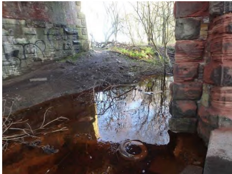
Figure 48 - Water ponding (under span 1)
