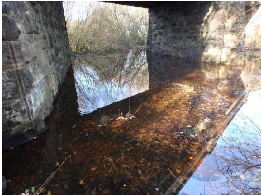
Figure 51 - Flooding under the structure in Nov 2019
