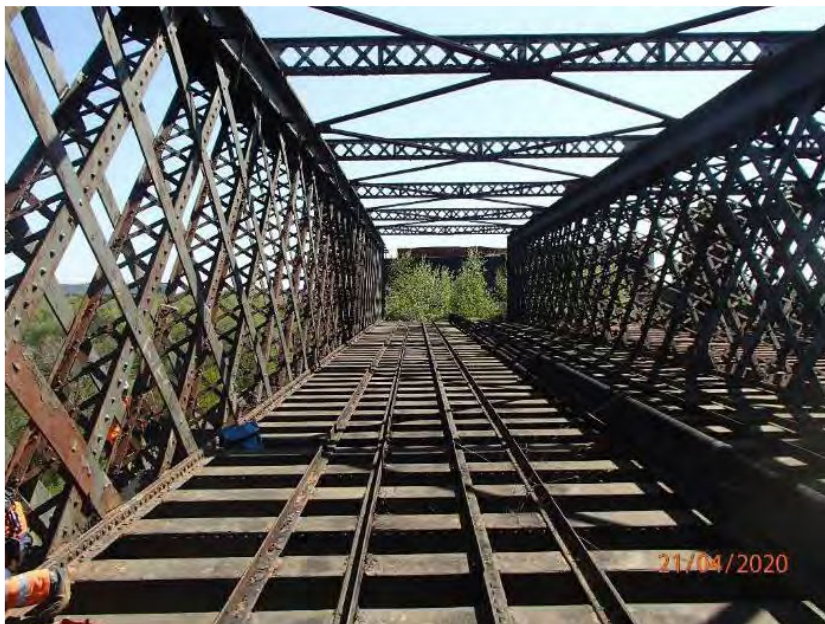
Figure 59 - Photo showing a view looking east along the northernmost deck showing the existing lattice girders and metal deck troughing
