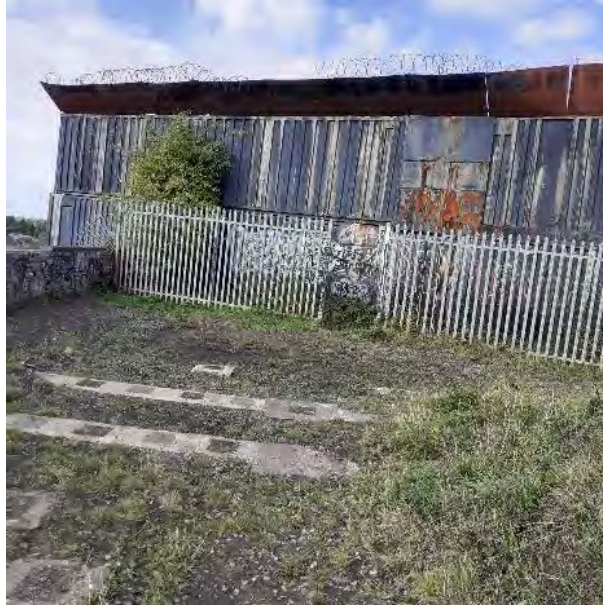
Figure 56 - Photo showing placement of shipping containers to prevent access to unsafe areas of the structure
