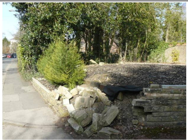
Photograph 26: Damaged Stone Boundary Wall and Tarmac Patch Repairs
