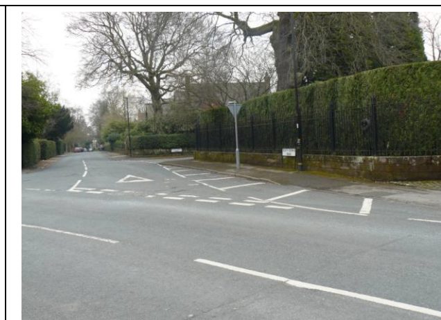
Photograph 28: Inappropriate Road Markings
