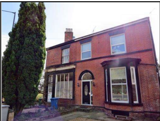
Photograph 140: Inappropriate Door and Windows, 33 Langham Road
