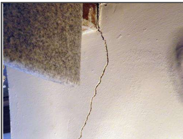
Photograph 143: Cracks in Plaster Reportedly Caused by Traffic, 7 Church Brow
