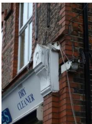
Rotten console to shop front where capping missing
