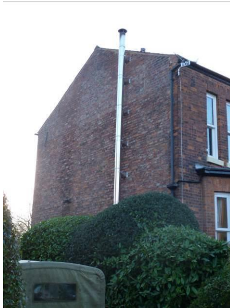
Unsuitable duct to gable wall of number 14
