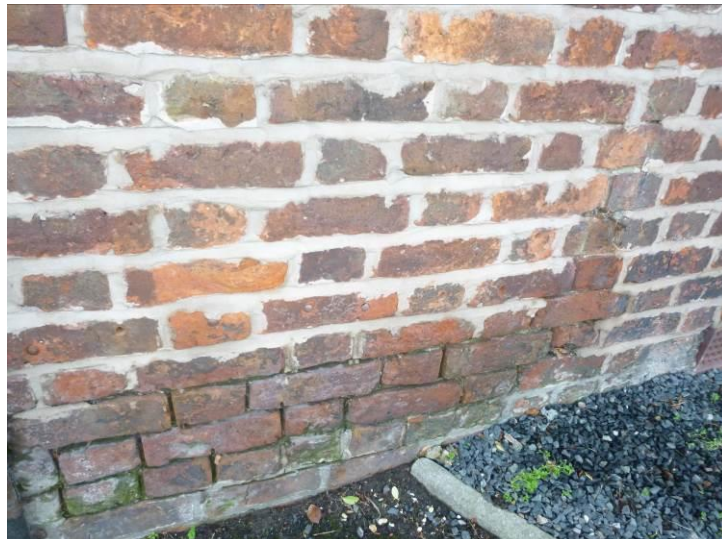
Hard cementitious pointing and eroded mortar
