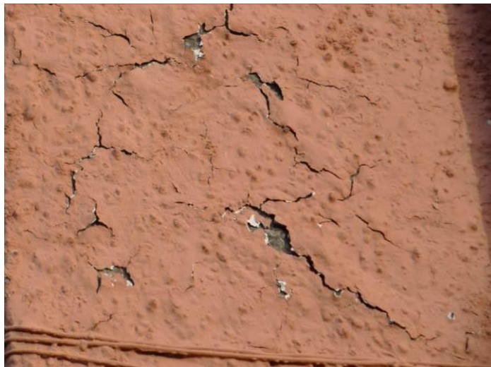
Cracked paint to roughcast render
