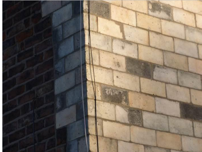
Damaged buff bricks to front elevation and hard cementitious pointing to gable
