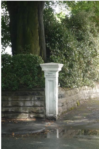
Original gate pier to North Woodville. This has been painted and is showing signs of erosion due to low level water damage.
