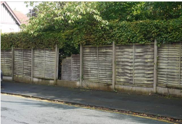
Timber panel fencing in Character Zone A that is inappropriate in style and in a poor condition
