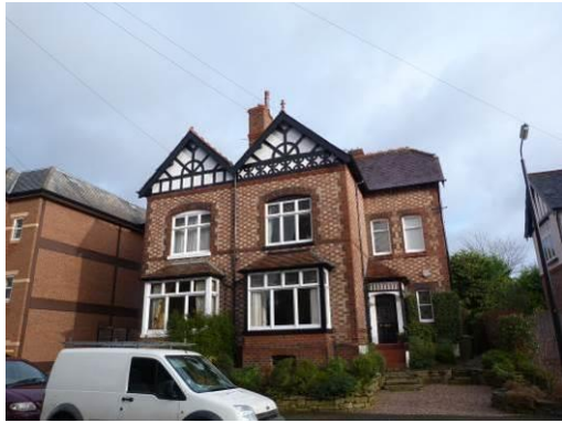
Polychromatic brickwork, rebuilt boundary treatment and a loss of decorative timber detail on the gable end
