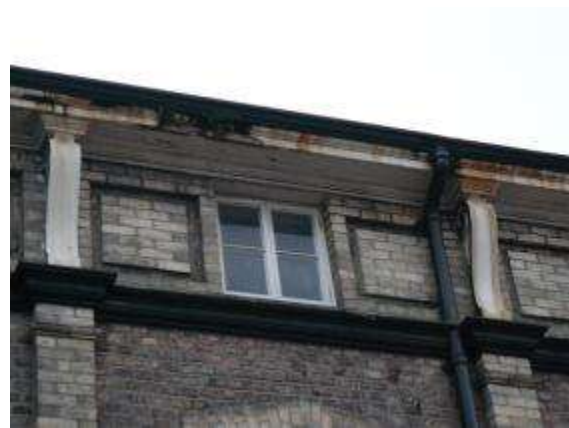
Photograph 23: Water damage to eaves No. 69 George Street
