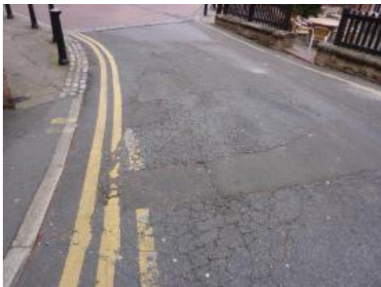
Photograph 44: Pooly maintained road surface on Denmark Street
