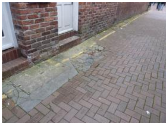
Photograph 45: Intrusive repairs to hard surfacing on Back Grafton Stree
