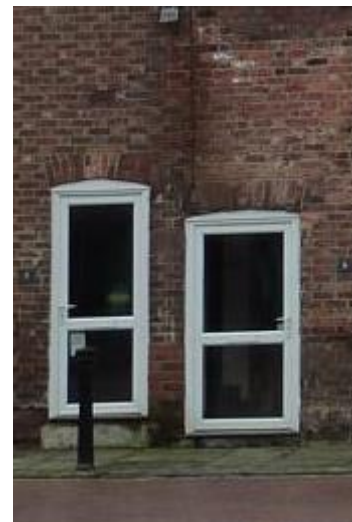
Photograph 20: Incongruous uPVC Doors to 5/6
