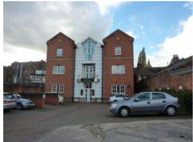
Photograph 96: Large area of deteriorating hard standing & tarmac to rear of properties on Church Street
