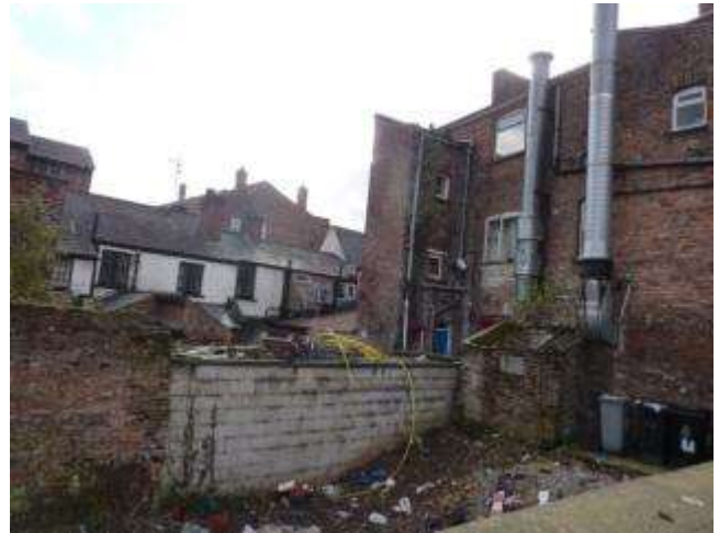
Photograph 86: Inappropriate siting of ventilation system
