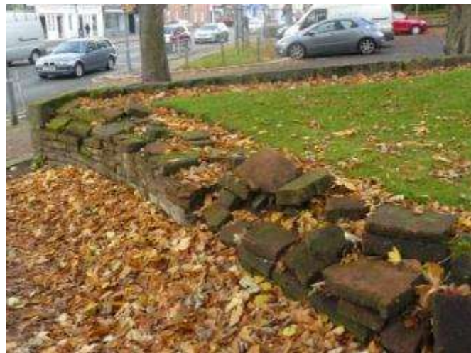
Photograph 92: Deteriorating stone wall adjacent to St George's Church
