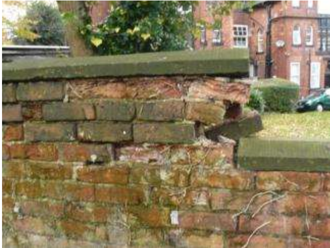
Photograph 93: Spalled brick boundary wall to Churchyard
