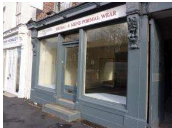
Photograph 29: Good example of a traditional painted timber shop front with vertically subdivided windows and centrally placed door mirroring symmetry on upper floors.
