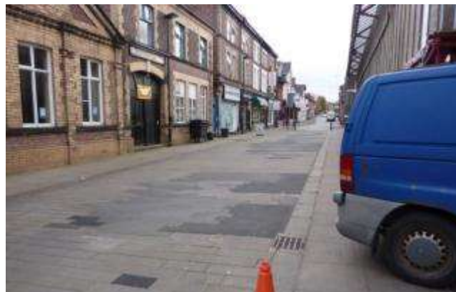
Photograph 98: Poorly repaired public realm on Greenwood Street
