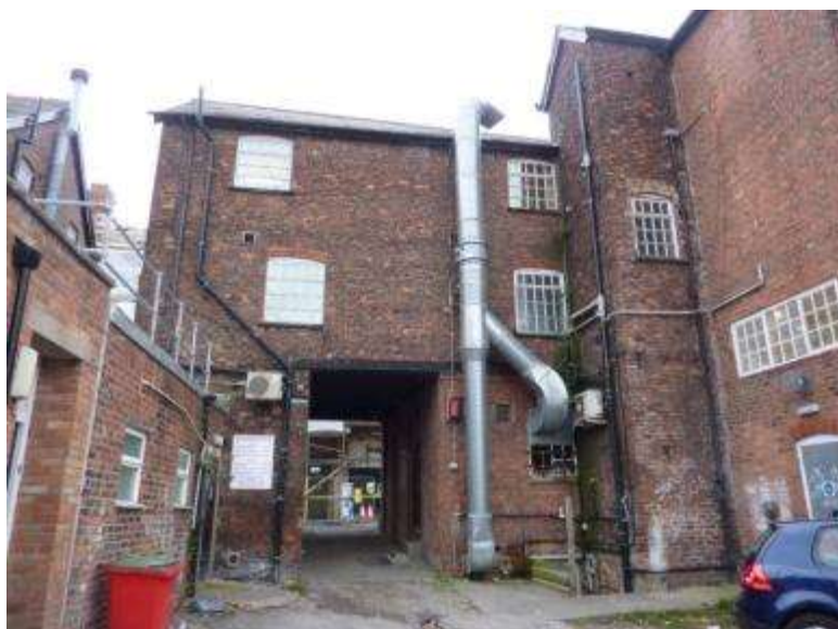
Photograph 36: Inappropriate siting of ventilation system
