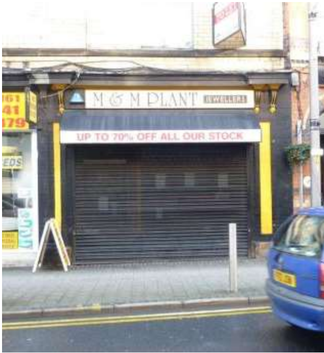
Photograph 21: Inappropriate signage, awning and roller shutters partially concealing original timber cornice, pilasters and corbels.
