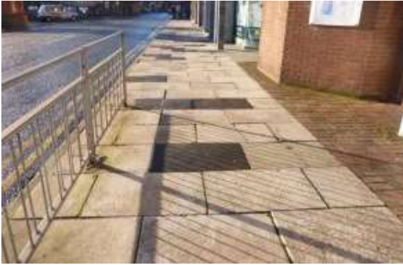
Photograph 25: Poor quality surface of paving slabs with areas of tarmac
