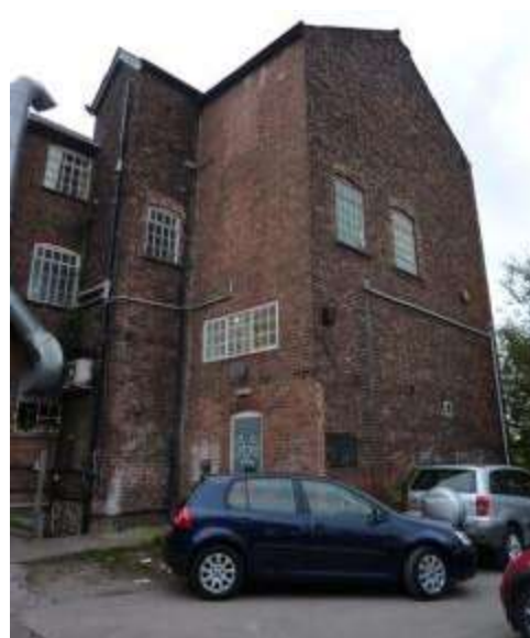
Photograph 37: Rear elevation of C.W Bonson's Store Rooms in poor condition
