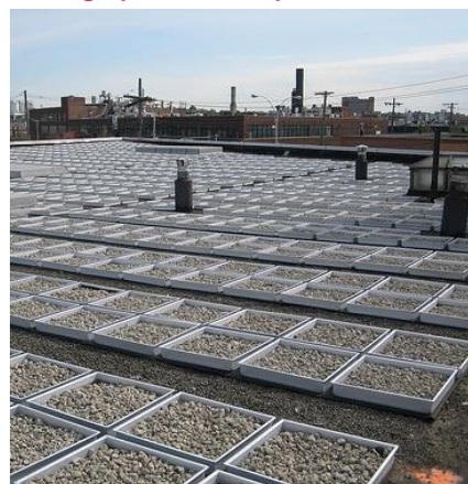
Photograph 47 - Example of a Blue Roof
