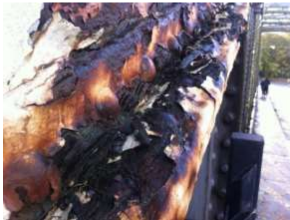
Extensive corrosion to the road bridge ironwork
