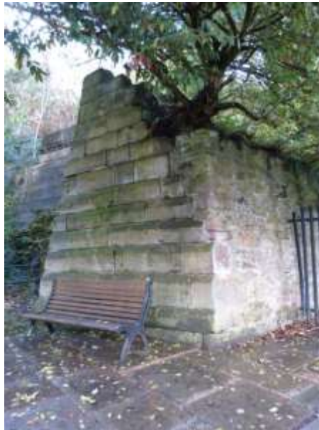
Self-seeded vegetation causing extensive damage to the former Brindley aqueduct on the north side of the canal
