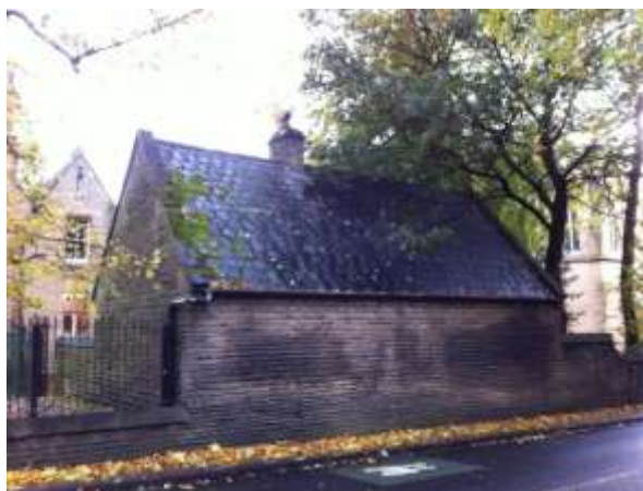
Moss build up due to overhanging tree to Presbytery outbuilding
