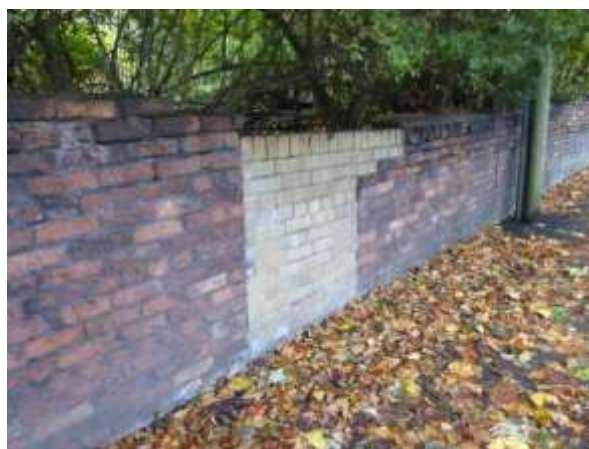
Boundary wall to Redclyffe Road showing unstable sections, eroded pointing and unsuitable repairs
