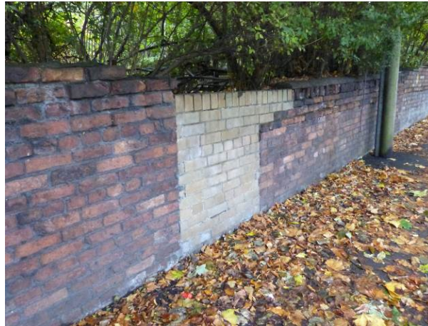
Inappropriate repairs to a historic brick boundary wall
