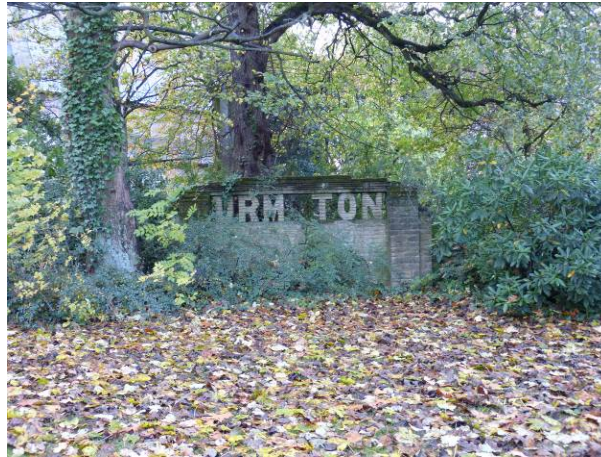
The Urmston sign, which is in need of repair
