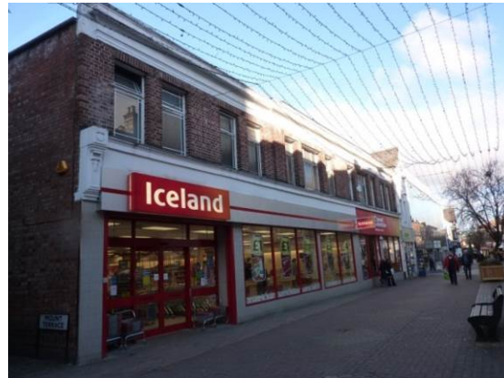
Nos. 88-90 George Street, which has a surviving historic corbel and classical parapet cornice
