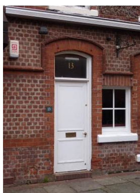
Thick, unattractive pointing at No. 13 Goose Green, where there is also evidence of spalling brickwork which is detracting from the otherwise attractive brickwork.
