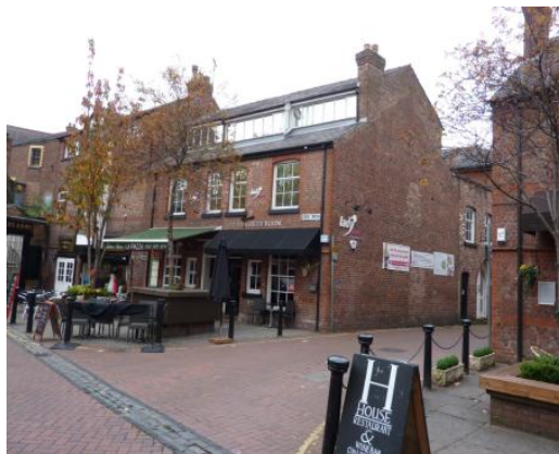
Inappropriate roof extension, Nos. 9 and 10 Goose Green
