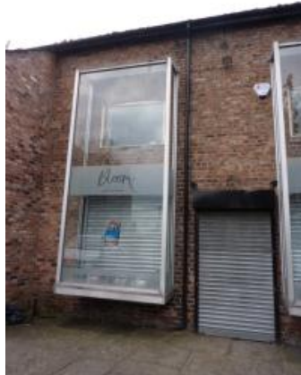
Inappropriate box windows, No. 7 Goose Green
