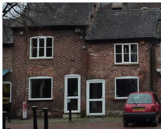
Inappropriate replacement doors and ground floor windows, Nos. 5-6 Goose Green
