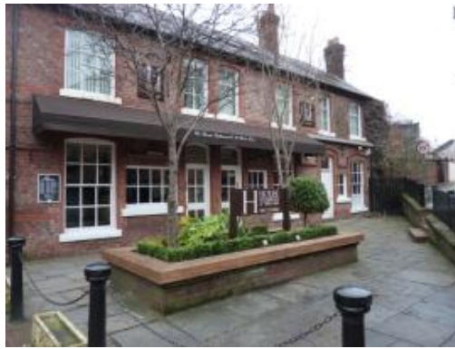
Nos. 11-13 Goose Green, which have lost their original architectural balance due to the addition of extra windows at ground floor level.
