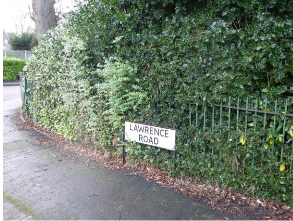
Historic railings in need of maintenance
