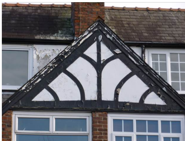
Imitation timberwork painted onto gable, in poor condition
