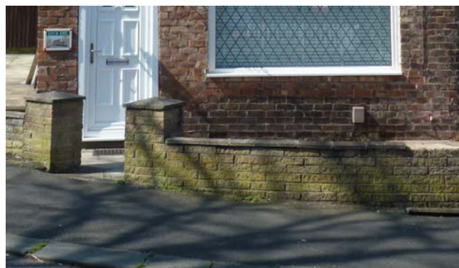
An inappropriate reconstituted stone wall to No. 72 Lock Road
