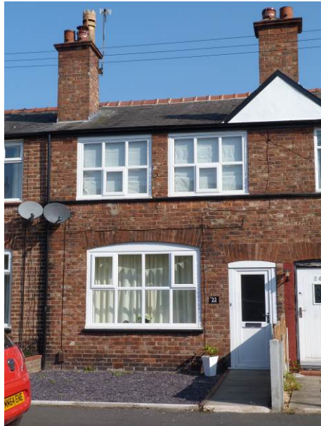
Inappropriate windows at No. 22 Place Road, which have the wrong frame composition. Note also how the top hung casements project outwards from the main frame, increasing the thickness of the frames and disrupting the smooth lines of the frame
