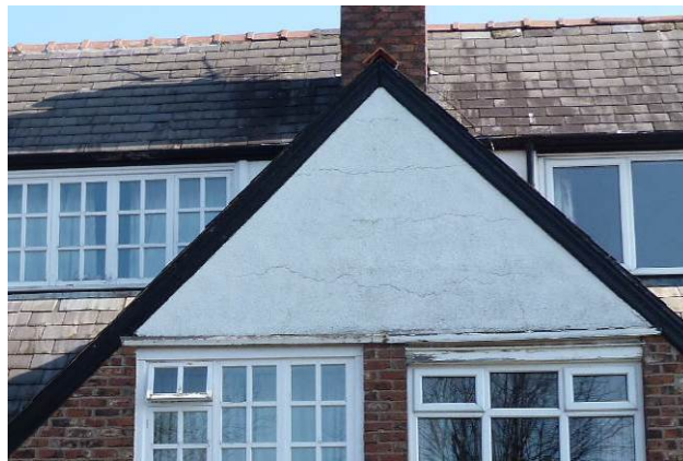
A gable which has lost its painted mock timber framing
