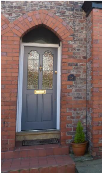
Door at No. 34 Weldon Road, which follows roughly the original design, using timber and glazed upper panels, but which does not exactly follow the original style and would therefore not be permitted in any future applications
