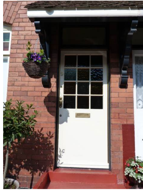
Original door to No. 9. Some of the coloured glazed panes have been replaced with textured glass
