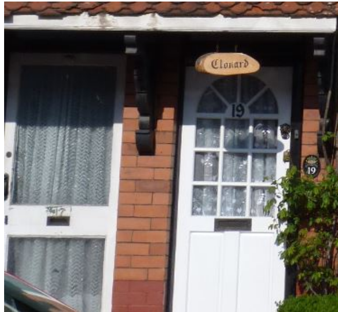
Inappropriate replacement doors to Nos. 17 and 19
