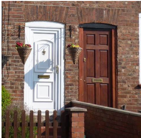
Inappropriate doors on Place Road
