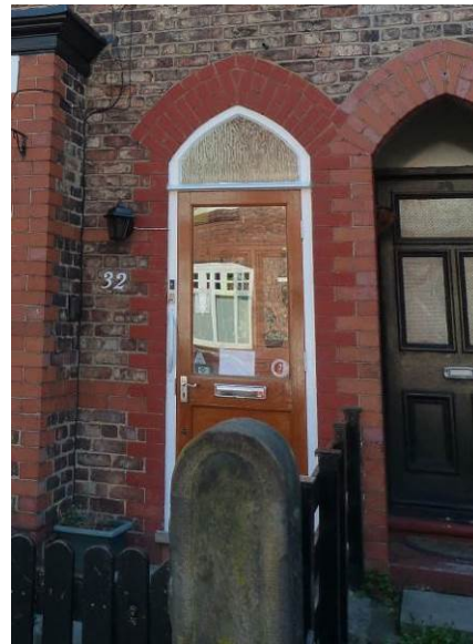
Inappropriate door at No. 32 Weldon Road in stained timber, which is set forward with the loss of the original porch
