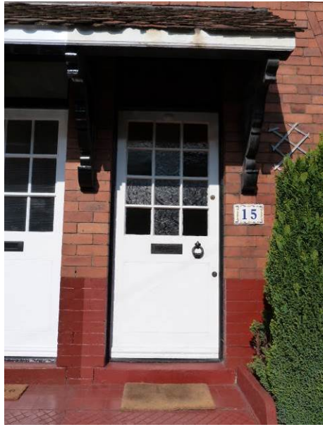
Original door to No. 15. Some of the coloured glazed panes have been replaced with textured glass
