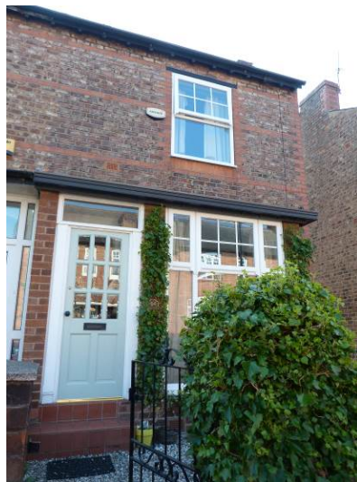
Inappropriate porch and uPVC windows at No. 46 Weldon Road
