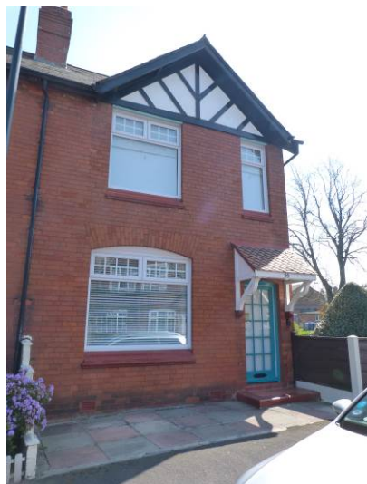
Style Six: Inappropriate windows and door to No. 55 Lock Road
