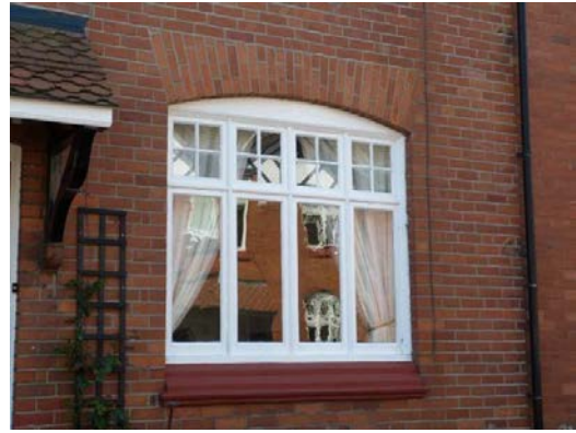
Style Six: Original window at No. 3 Pollen Road, though this example has lost its coloured glass
