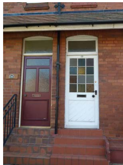
Style seven: An original door to No.17 Norman Road (right) and a replacement door to No.15 Norman Road (left)
