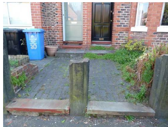
Original diamond pattern textured paving to Nos. 18 and 20 Weldon Road, together with damaged original stone gateposts
