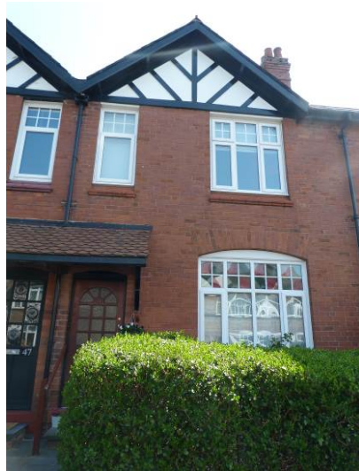
Style Six: uPVC examples of windows following the original design, though with bulkier frames
