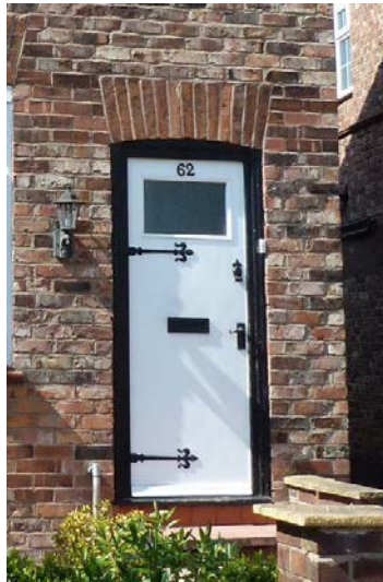
Original door at No. 62 Lock Road, though the decorative ironwork is not original and is inappropriate
