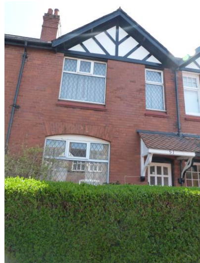
Style Six: Inappropriate leaded windows at No. 51 Lock Road
