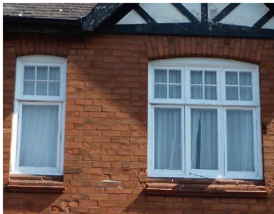
Style Six: First floor windows to No. 59 Lock Road showing side hung casements to lower panes
