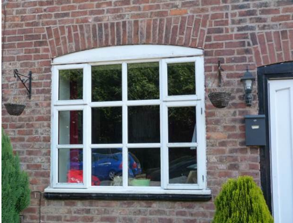
Inappropriate windows at No. 107 Lawrence Road
