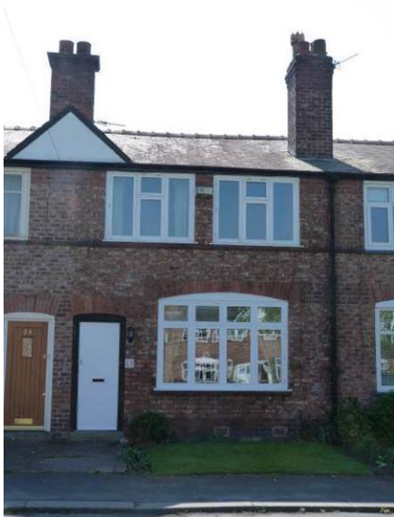
Replacement timber windows at No. 25 Bemrose Avenue. These are timber frames. The ground floor window has the correct frame design but the first floor windows lack some of the smaller upper panes. The frames are also thicker than the original examples
