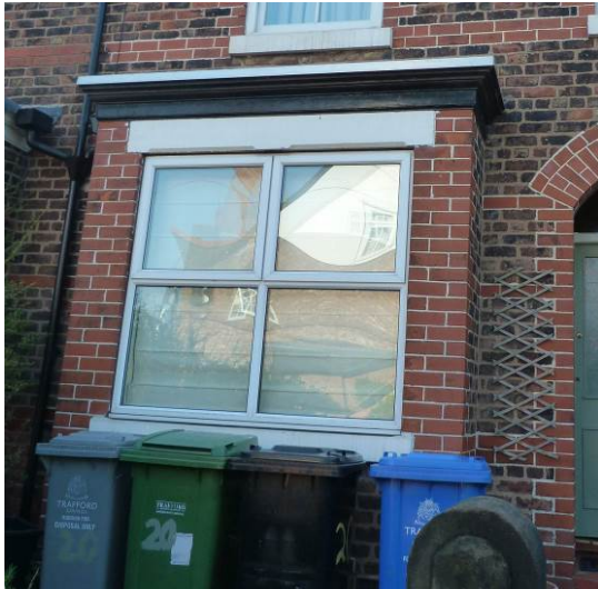
Inappropriate uPVC windows to No. 20 Weldon Road
