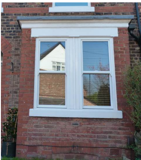
uPVC sash windows to No.22 Weldon Road in an appropriate design mirroring the original timber versions
