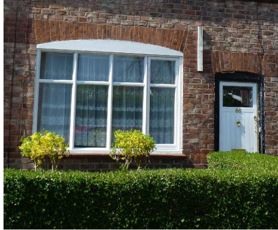
Detail of original window (note side hung casement to the side of the window nearest the door) and door at No. 66 Lock Road
