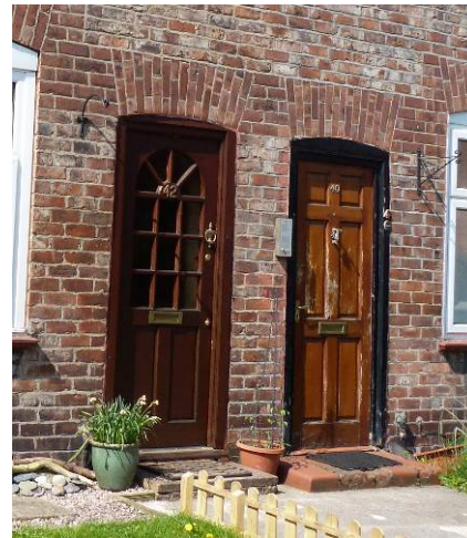
Inappropriate doors on Lock Road
