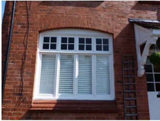
Style Six: Original window featuring coloured glass panes on No. 57 Lock Road
