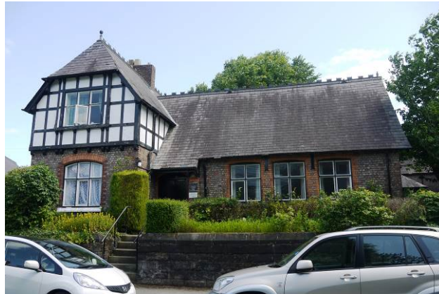
Unitarian Church Hall, Sylvan Grove requires some maintenance
