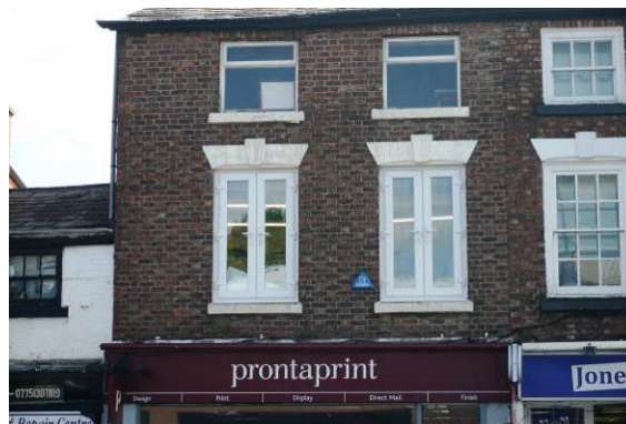
Unsuitable materials and designs used on replacement windows along Church Street
