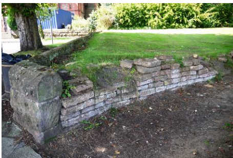
Boundary wall to Church of St George in a poor condition
