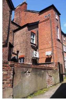
Poor condition of boundary treatments and rear elevations
