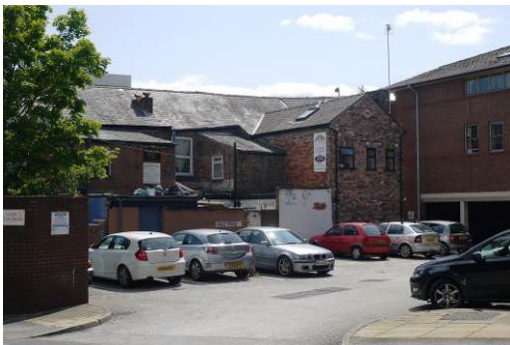
Rear elevations are often neglected and are deteriorating
