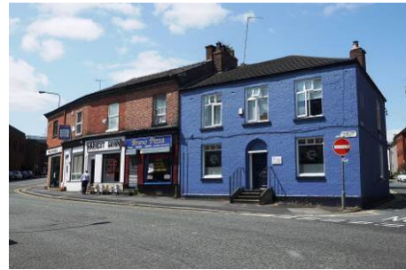
Inappropriate painted brickwork on Stamford Street
