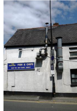
Intrusive ducting and, ventilation inappropriate render in a poor condition and modern signage
