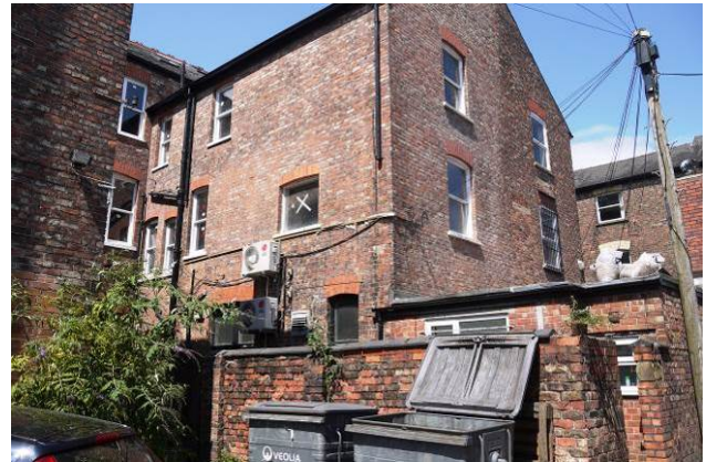
Typical issues to the rear of properties including vegetation growth, air-conditioning units, bins and brickwork in poor condition.
