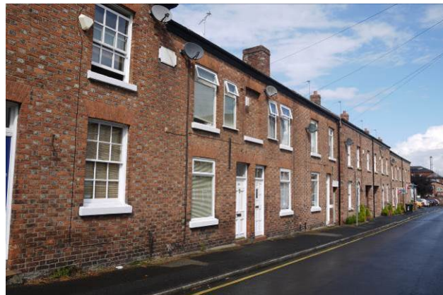
Simple terraces on New Street harmed by inappropriate style sash doors, uPVC windows and intrusive satellite dishes
