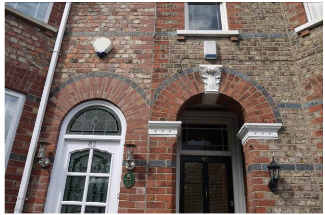
Additions to the ends of terraces attempt to emulate the existing structures but fall short on detailing such as decorative key stones and corbels
