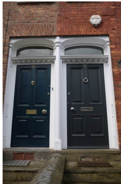
Original door on the left and a replacement on the right at Nos. 72-74 New Street
