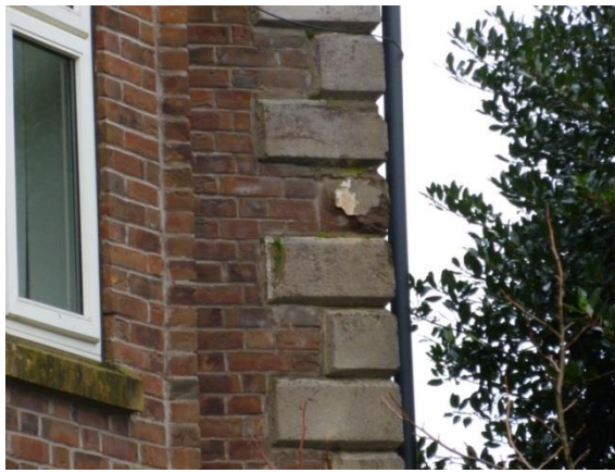
Delaminated stone quoin to Old Hall Farmhouse
