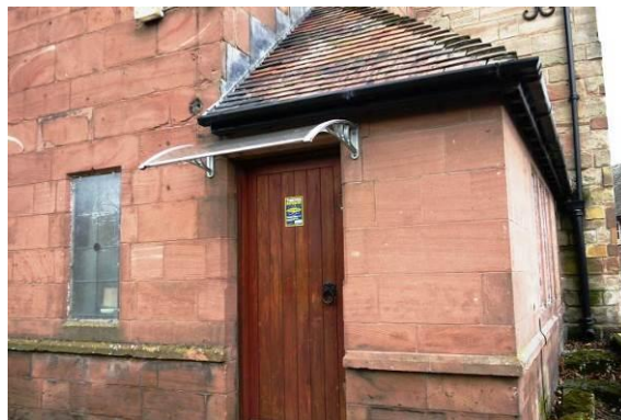
Inappropriate detailing on the church
