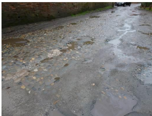
Uneven and partially covered stone sett surface
