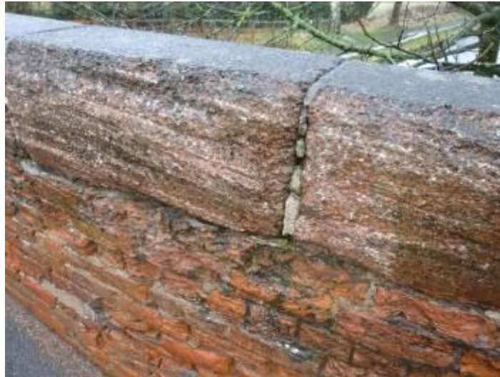
Eroded concrete copings and spalled brickwork below
