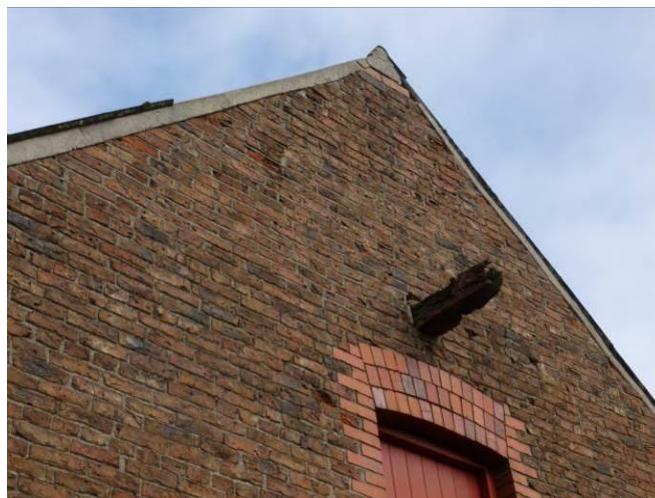
Lifting Beam to Ash Farm barn, missing roof sheet above
