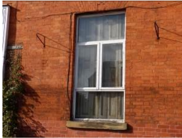
An example of the distinctive timber-framed windows on Cornbrook Terrace. Note the timber shutters on the inside.
