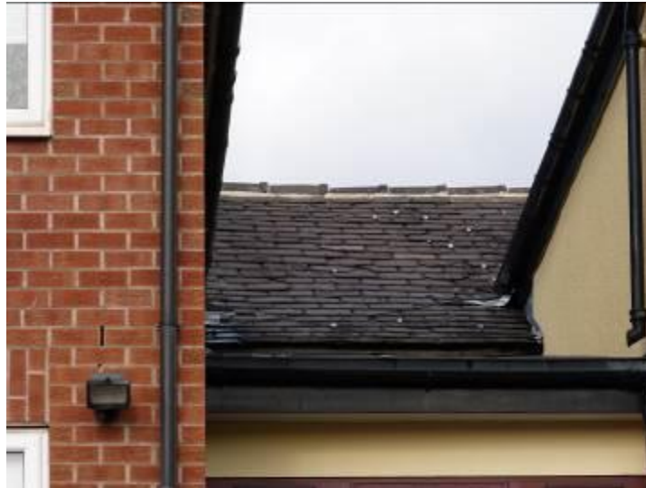
Cracked and slipped slates to rear roof slope, visible between modern extensions
