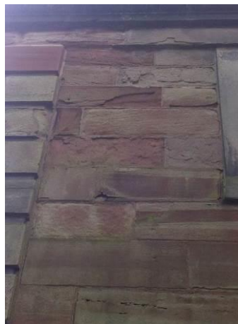
Delaminated sandstone to church walls
