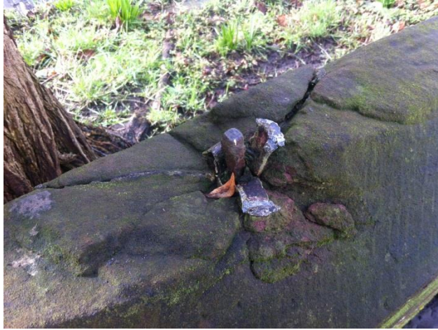
Damage to church wall copings from former railing fixings
