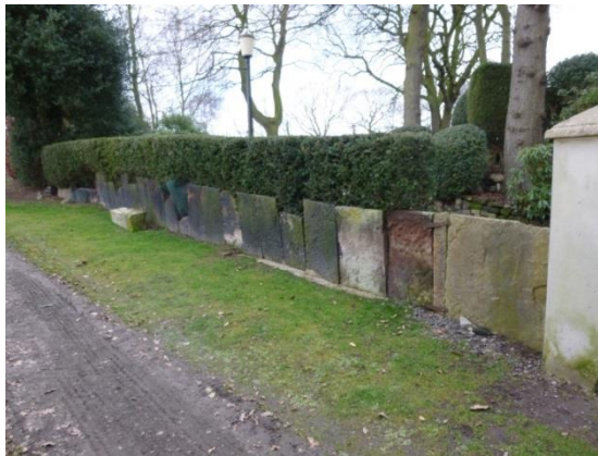
Vertical sandstone flag boundary wall to rectory, with multiple fractured flags
