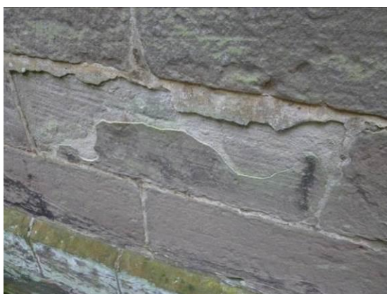
Example of delamination to ashlar on St. Werburgh's Church
