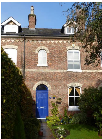
An original ground floor window at No. 12 Brogden Terrace, with later replacements on the upper floors.
