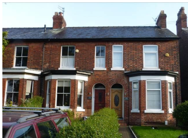
Inappropriate replacement windows at No. 23 Brogden Grove, with transoms which disrupt the rhythm of the wider terrace's fenestration.
