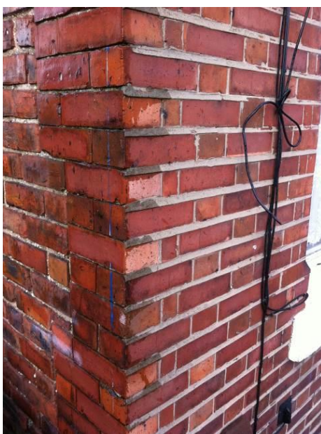
Damaging cementitious ribbon pointing.
