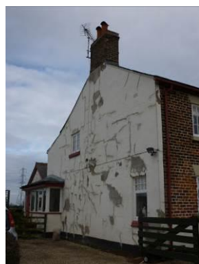
Failing and poorly-patched render on Bollin Cottages
