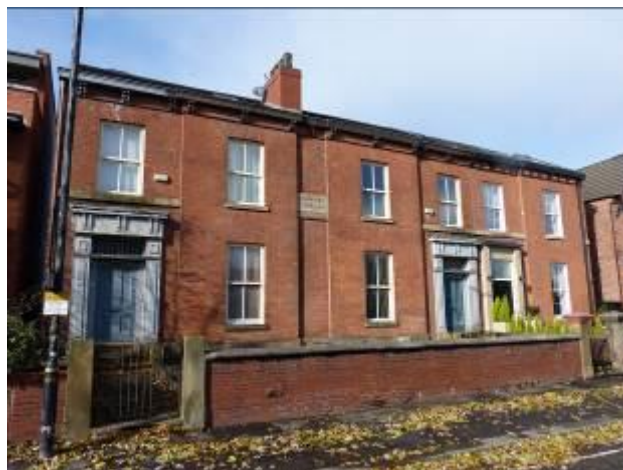
Chester Terrace, with original doors and windows on the left and in the centre, and unsympathetic replacement door and windows on the far right
