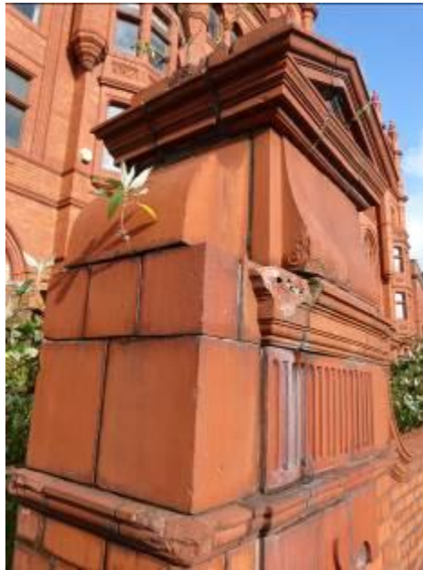
Damaged terracotta detailing to the front boundary wall of the Essence Factory
