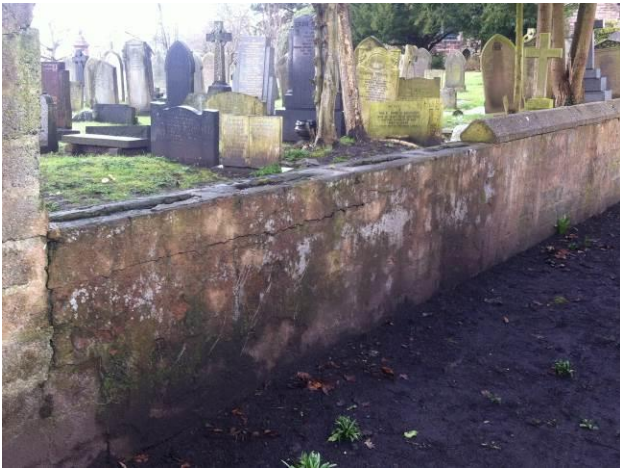
The historic stone boundary wall to the church is in a poor condition in places; it has been rendered and coping stones have been removed
