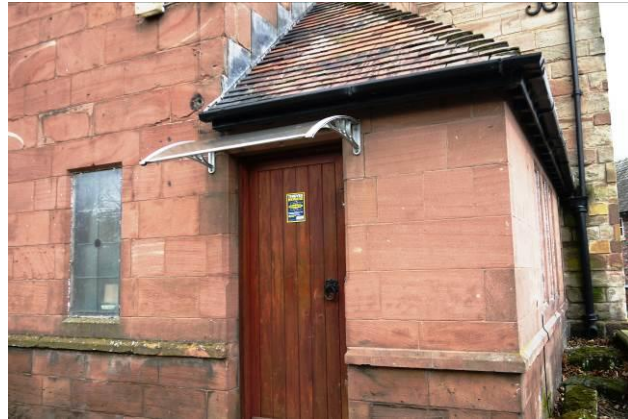
Inappropriate modern porch projection
