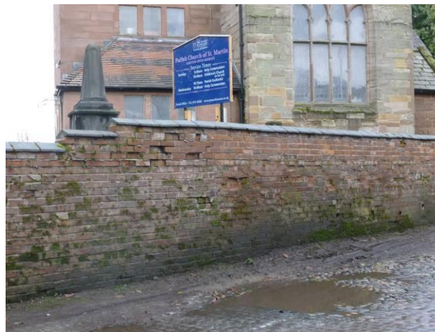
Church boundary wall in need of some repairs and repointing
