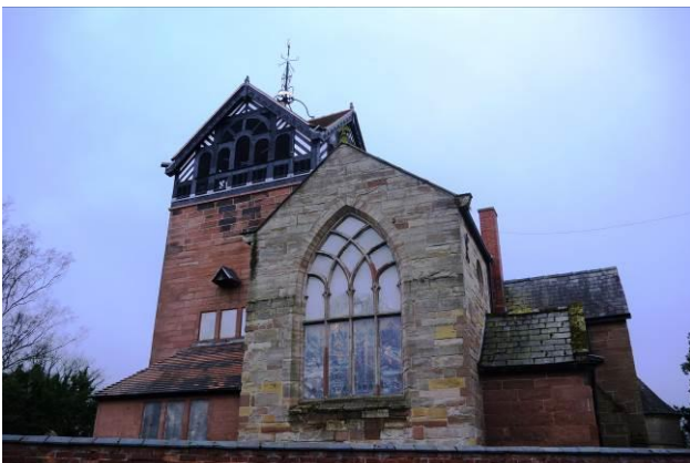
Intrusive polycarbonate protective glazing to the east window of St Martin's Church
