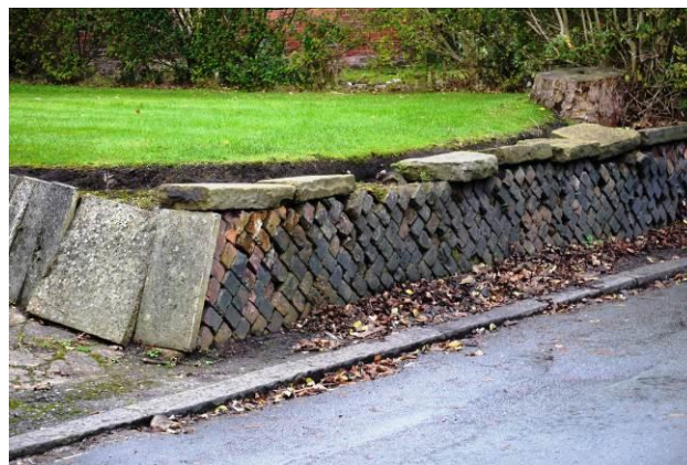
Herringbone brick boundary wall, in a poor condition
