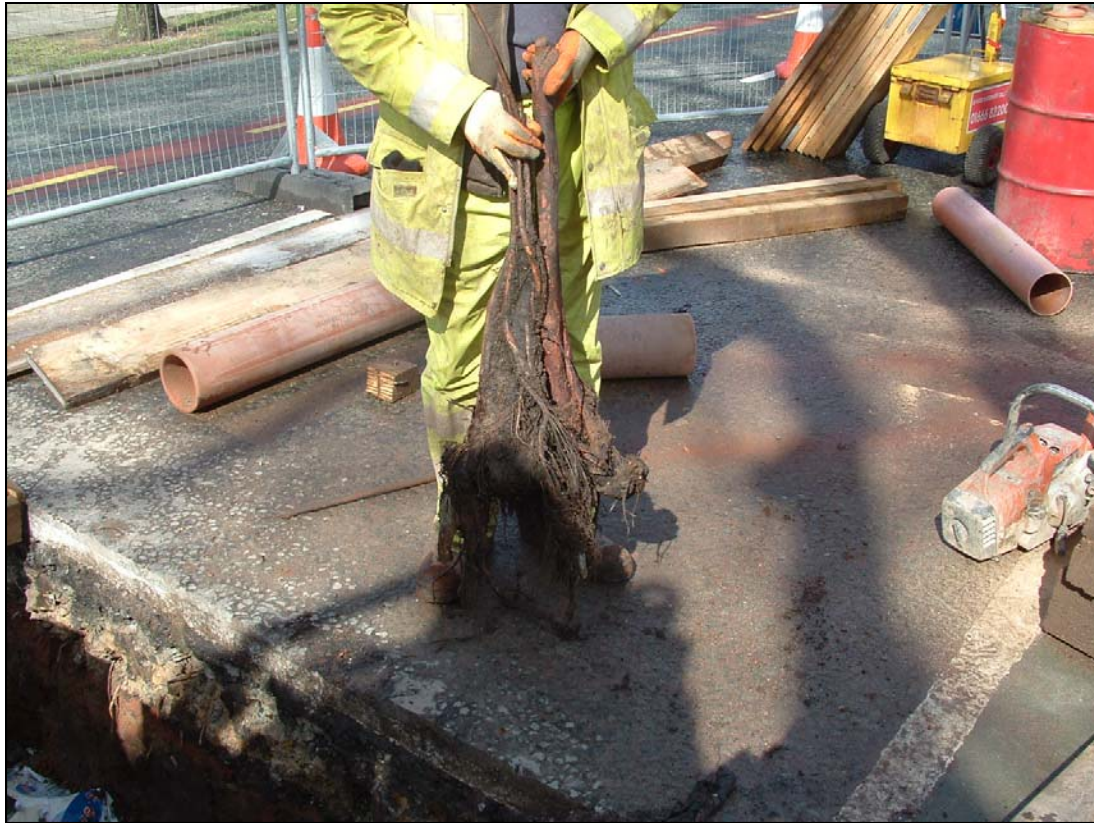
Photo 2 - result - tree root blocking highway connection to the sewer, approximately 8 metres in depth
