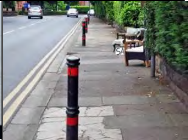
Photograph 28: Bollards, Cracked Flagstones and Yellow Lines (Ashley Road)
