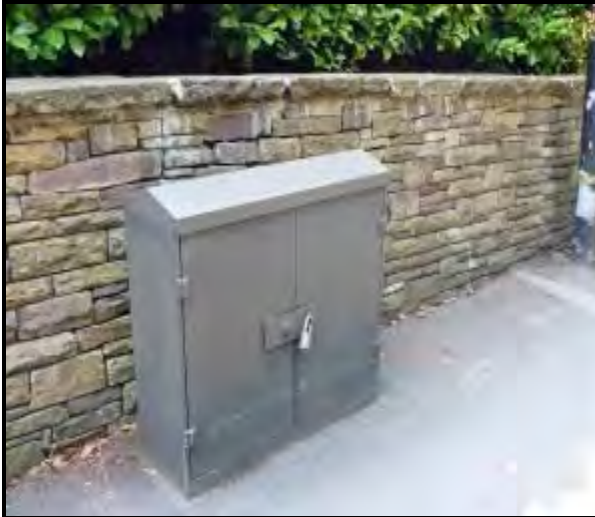
Photograph 78: Services Cabinet on Hale Road
