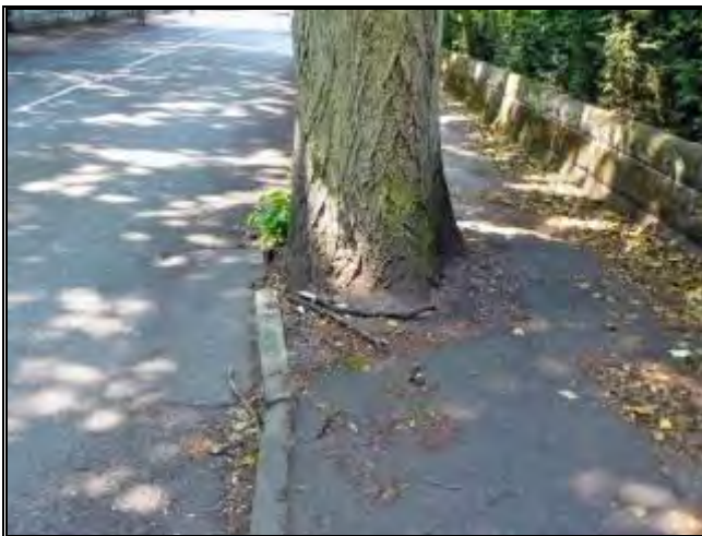
Photograph 125: Root Damage to Curbs, Harrop Road
